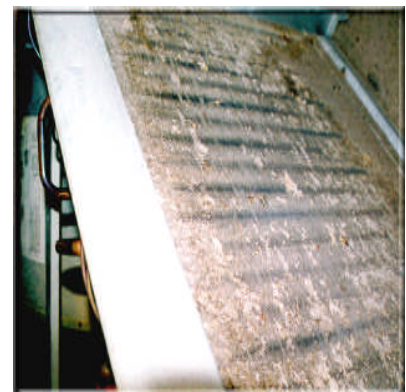
Typical A/C e-coil loaded with mold growth and debris
